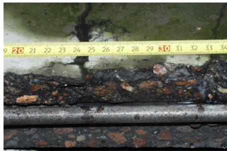
Corrosion at 24, 33 cm
